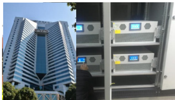
Guangzhou Telecom Building AHF&SVG
