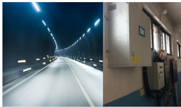
Hangzhou Ring Expressway Tunnel AHF
