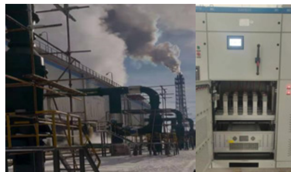
■ CNOOC Hegang Self-Owned Power Plant SVG
