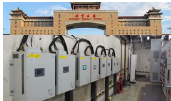
Beijing West Railway Station AHF
