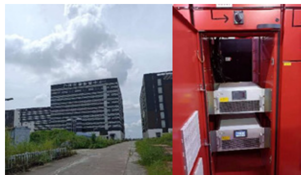
Guangzhou Big Data Center AHF&SVG
